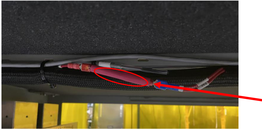
Figure 12-9 – #14 Thermal Fuse (Engine Room)
